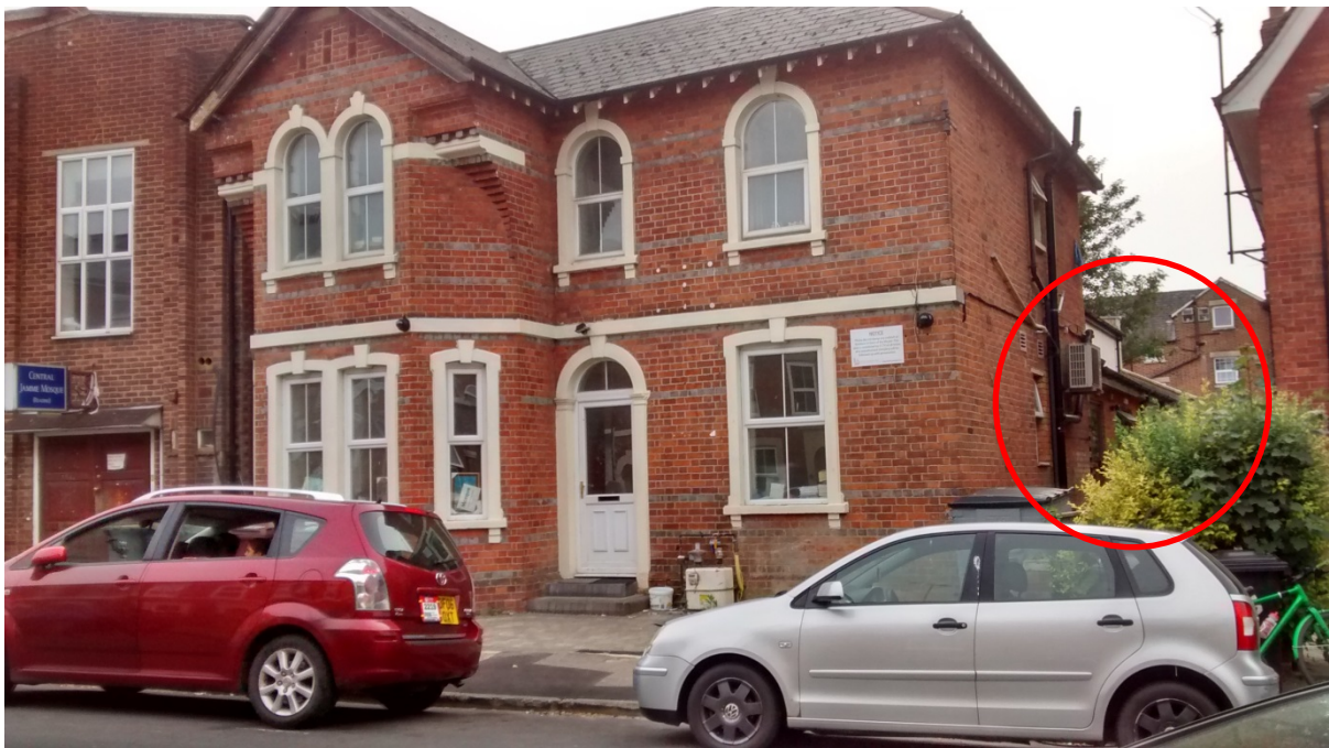
Site in current view from Waylen Street. Unauthorised extension is just visible in the red circle. Front boundary wall is missing.
